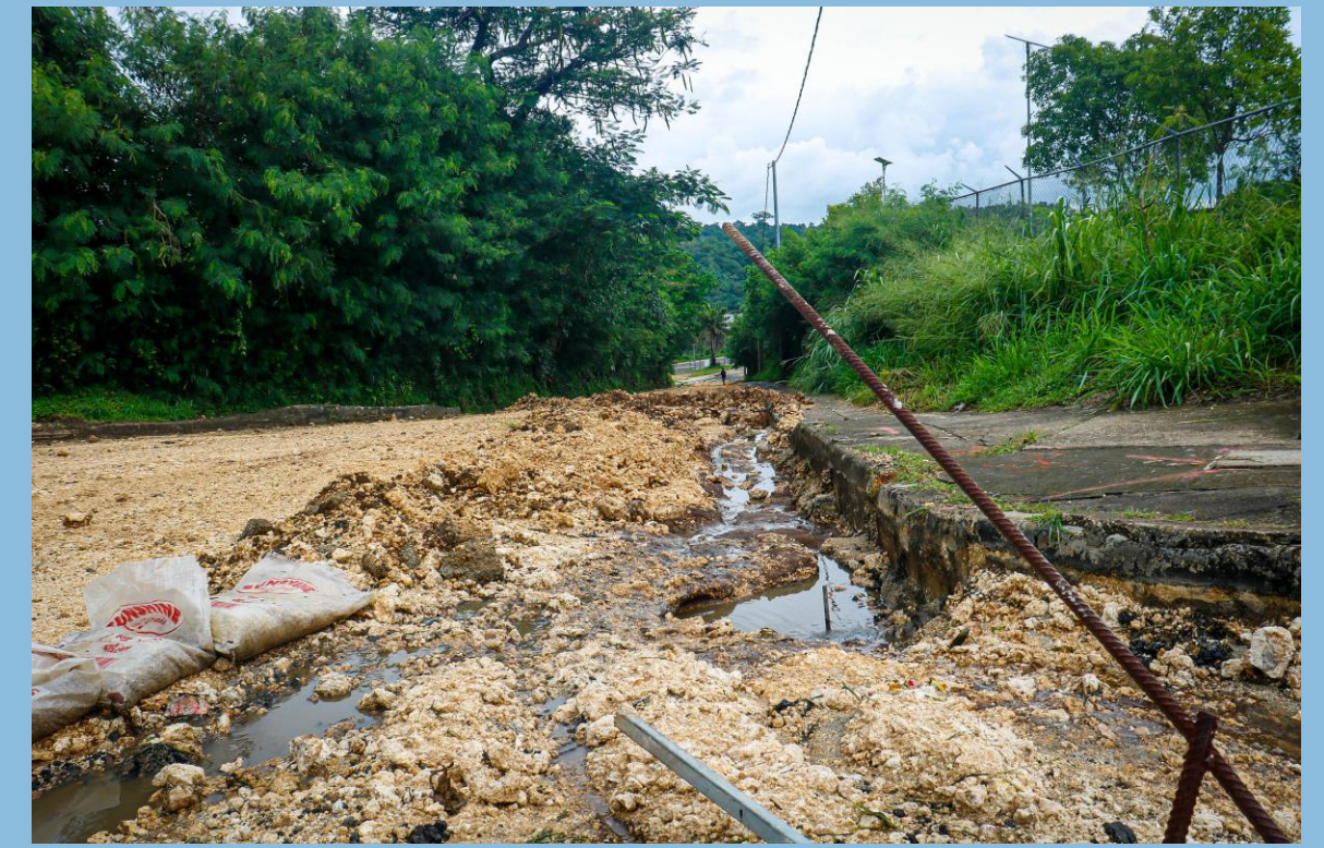
It started out as a pothole ! (VTU)
